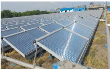
Fig 1: Solar Desalination Plant installed at NTECL
